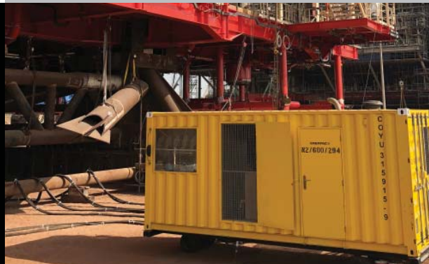
Enerpac Self-Propelled Power Pack that powered the ‘Push-Pull’ system for the platform load-out.
